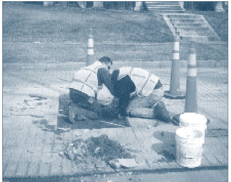
There are unique challenges involved in preserving historic roads. In Duluth, Minnesota, citizen activists are working to save their granitoid streets. Granitoid was an innovative concrete pavement (installed 1909-1910) designed to serve both automobiles and horses.
